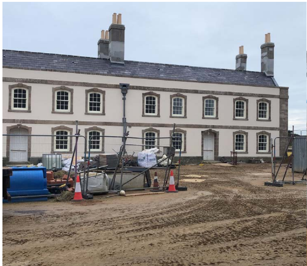
Jersey Heritage: The Officers' Quarters on the Parade at Elizabeth Castle is being renovated to provide group accommodation
